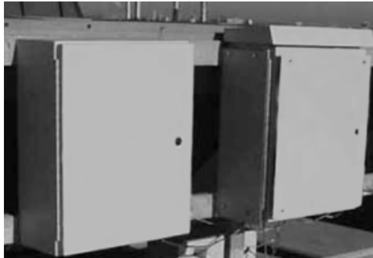
A test to compare the shielding effect on internal temperature rise was performed on similar enclosures exposed to the sun. The enclosures are the same color (RAL 7035 light gray) and material. The enclosure on the left is unshielded, the enclosure on the right is shielded on top and applicable sides.
