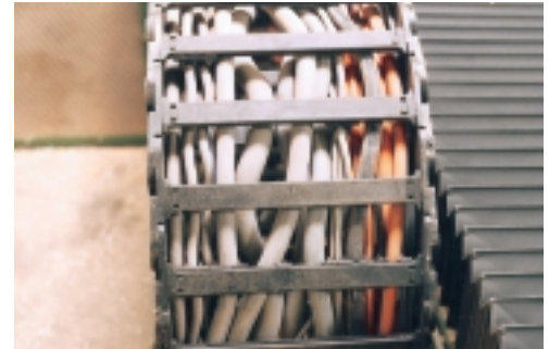
Corkscrewing: an effect of improper cable and hose placement in an Energy Chain®
